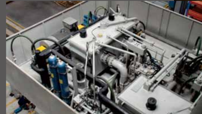
3D simulated arrangement to having clean and neat pipe / cable arrangement for the best space utilization
